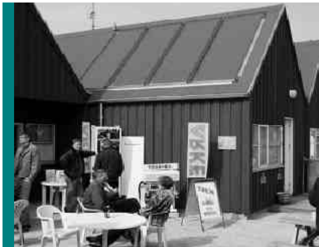
Maarup port: Solar heating plant at the harbour of Maarup, Samsø.
