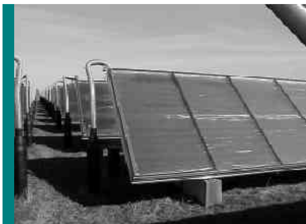
Aero-wvc: Solar panels of the 9,000 m 2 solar heating plant in Marstal, Ærø.
