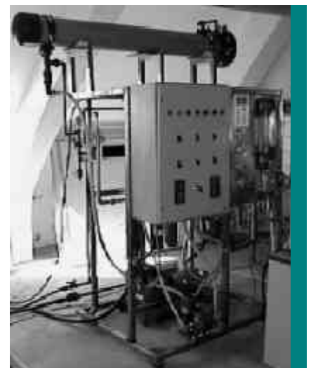
Fig 12: RO desalination plant (3 m 3 /d)
