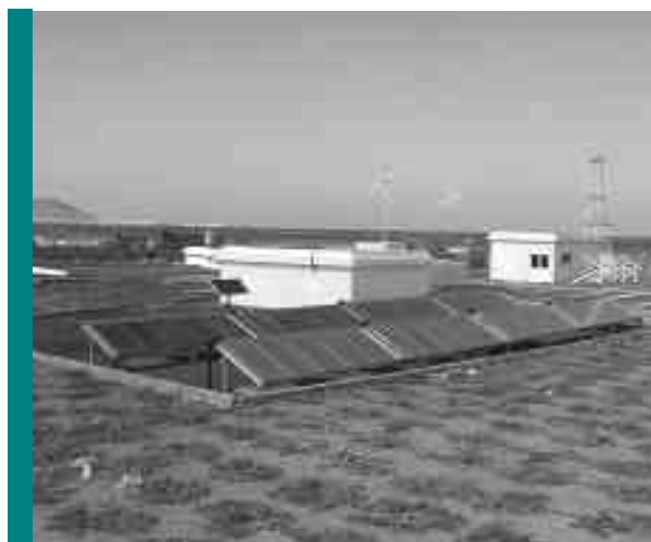
Fig 13: View of the solar thermal field (50 m²)
