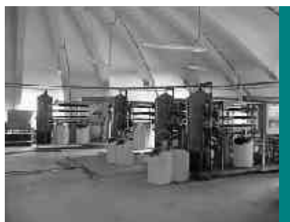
Fig 3 View of the Reverse Osmosis units
