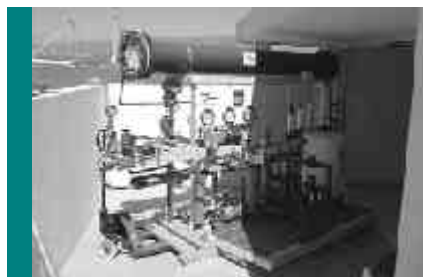
Fig 10: View of the reverse osmosis plant (18 m 3 /d)
